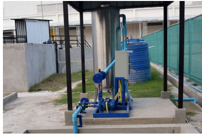
Wastewater treatment system at Nikon Lao Co., Ltd.
