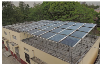
Solar-powered water heater at Hikari Glass (Changzhou) Optics Co, Ltd.
