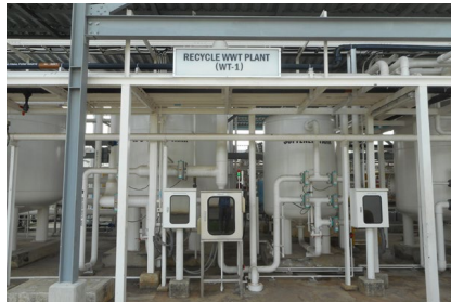
Wastewater processing plant at Nikon (Thailand) Co., Ltd.
