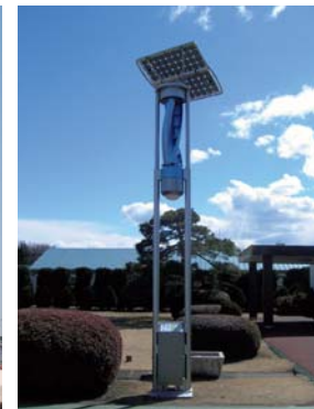
Lighting system that uses wind & solar power
