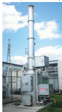
Gasification furnace (Sendai Nikon)
